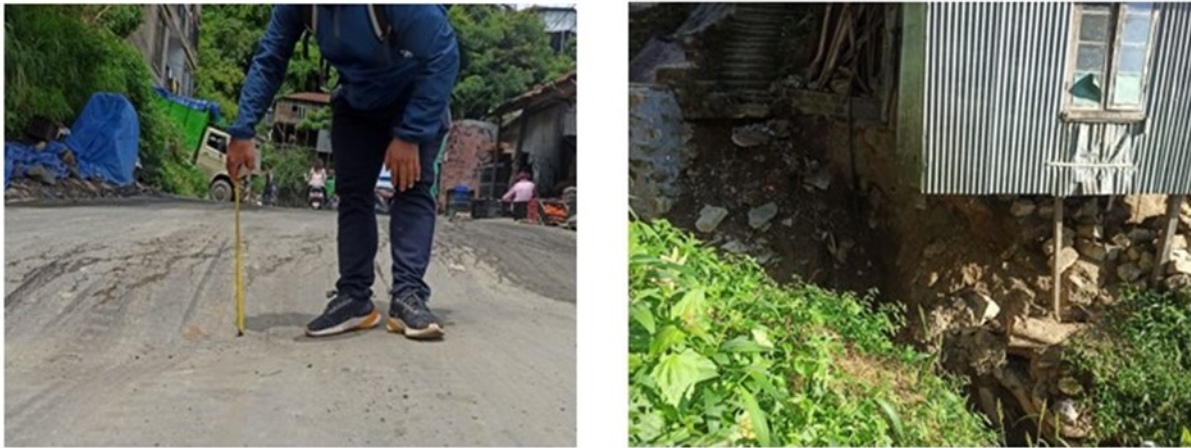
Figure 1: Field photographs of ground displacement at Zuangtui Area
