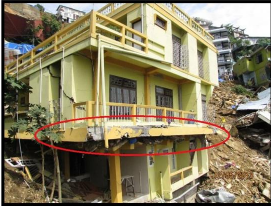
Figure 4. Marked line indicated one storey failure of the affected residential at the toe region.
